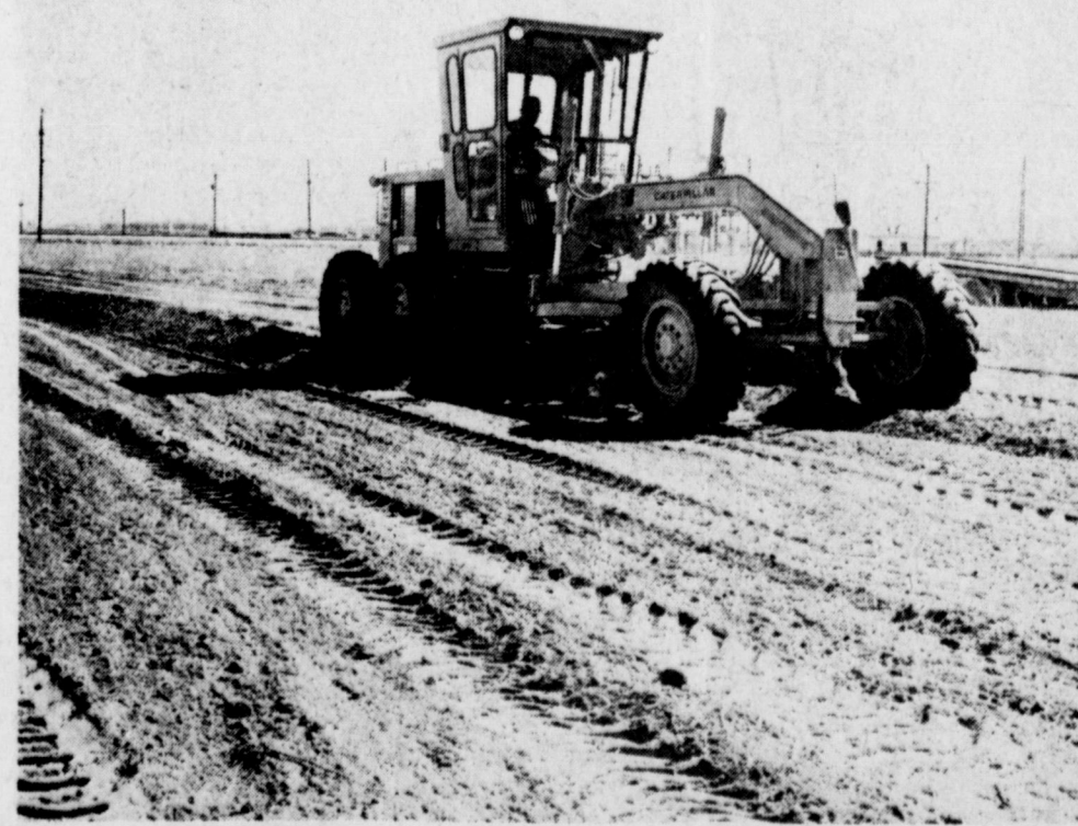
LAND LEVELING STARTS...Elmo Owen, occupying the maintainer started leveling land where a miniature golf course will be constructed by the Muleshoe Youth Activities Committee. The golf course will be constructed just to the east side of the Bailey County Exhibition Center and Coliseum on land contributed by the Bailey County Commissioners Court.
