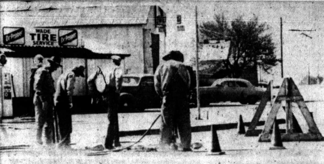
INSTALLATION WORK was begun today on the new traffic signal light at the intersection of Foster and North Hobart. Preparatory work should take about four days, according to Fred Brooks, acting director of Public Works. (News Photo)
