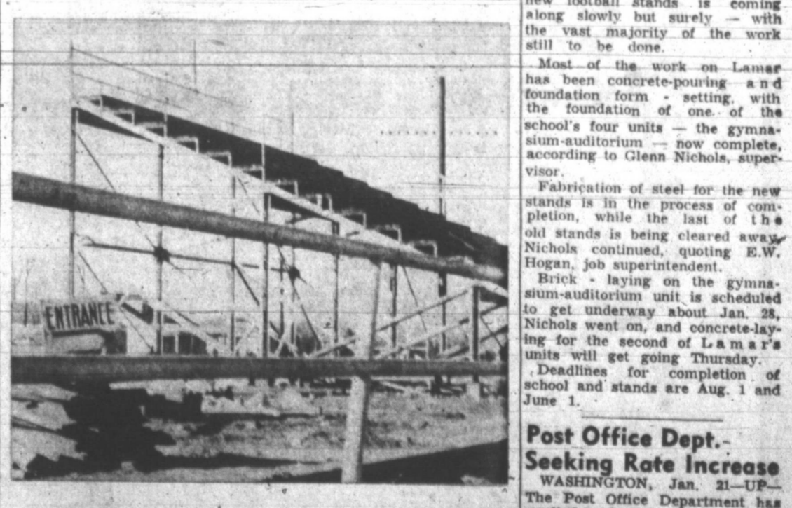
ENTRANCE TO WHAT? — Work on the new football stands on the west side of Harvester Park is coming along — but, so far, in a negative direction. Pictured here is the only portion of stands still standing, the rest of them (foreground) having been pretty much cleared away. The sign serves only to indicate that the new stands will be on this site, come September. (News Photo)
