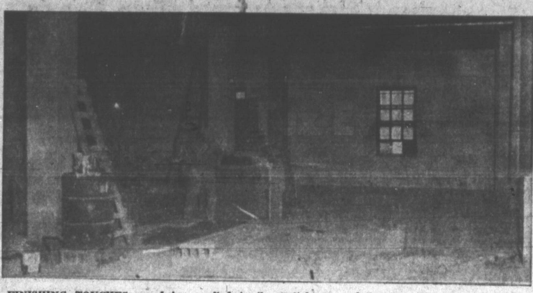
FINISHING TOUCHES are being applied to the switch room of the almost completed annex to the Southwestern Bell Telephone Co. building here. Pictured above is the large room where soon will be filling up the emptiness with intricate dial system equipment. The trimming, painting, and dressing up of the building should be finished in about 10 to 15 days so it will be ready when installation starts on May 4. (New Photo)
