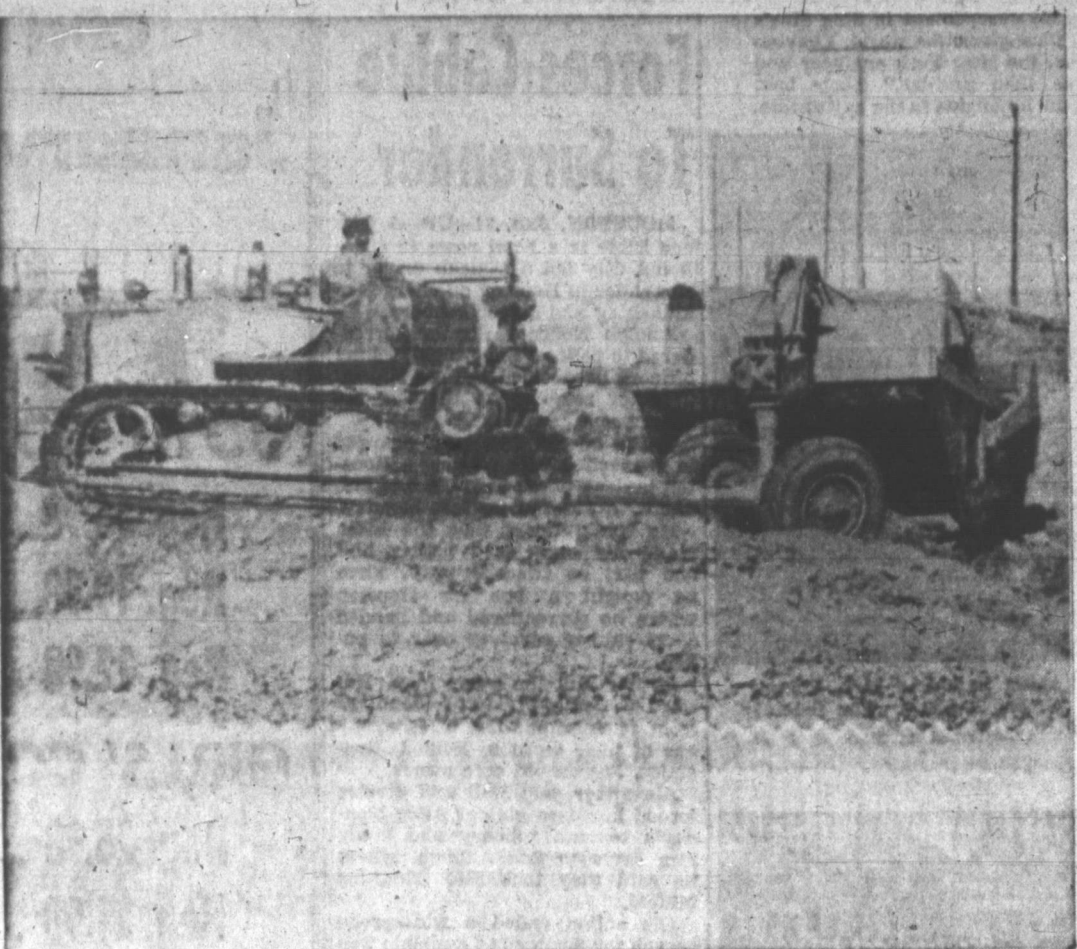
WORK PROGRESSES on the county road leading to Perry LeFors Field northwest of the city. Pictured above is road building machinery of Orville Thornburg Jr., dirt contractor on the paving job that will eventually provide an all-weather, hard-top road to the county's airport. (News Photo)
