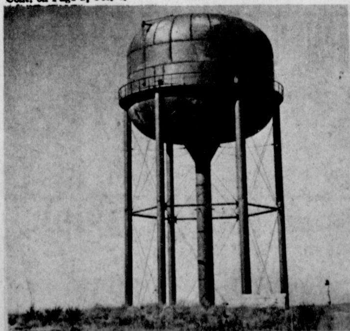
WAITING FOR A PAINT JOB . . . The City of Muleshoe is just waiting for the sub-contractors to come in and paint the new tank. It lacks cathodic protection and some electrical work.
