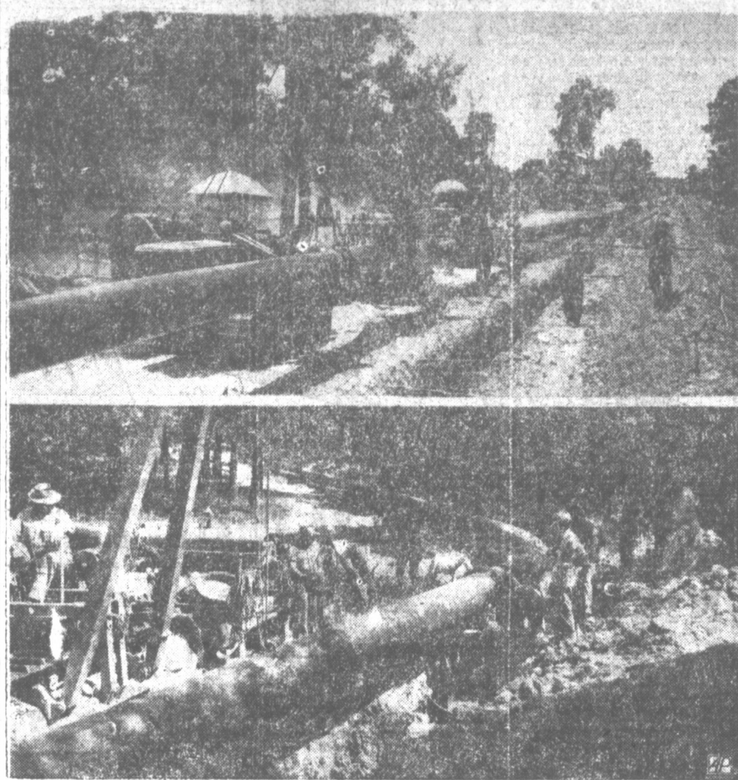
Construction work on parts of the $54,000,000 gas pipe line from the Corpus Christi area to West Virginia is shown near Houston (top photo) and near Huntington, W. Va. (lower photo). The line will start feeding 287,000,000 cubic feet of Texas gas daily to war industries in the Appalachian sector about Oct. 15, according to Gardiner Symonds, president of the Tennessee Gas and Transmission Co. (AP) Photo.
