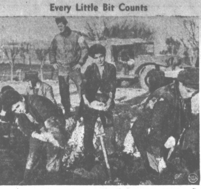
Every Little Bit Counts With small, but willing hands, these Italian youngsters, do a man-sized job of repairing roads in Italy. Volunteers all, paid regular wages by U. S. government, they're pictured working under supervision of Sgt. Joe Scydowski (rear) of New Britain, Conn.
