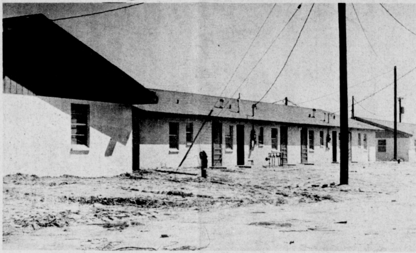
CONSTRUCTION CONTINUING...Construction is still underway on the Agriculture Housing complex on East Sixth Street in Muleshoe. Many of the units are nearing completion, although the overall project is still under construction. The cinder block housing units will be occupied by agriculture workers on completion, with a target date for completion possible late in November. Paving has been added, providing easier access to the units. Nearly 50 units are under construction, featuring two and three bedroom housing units for families.
