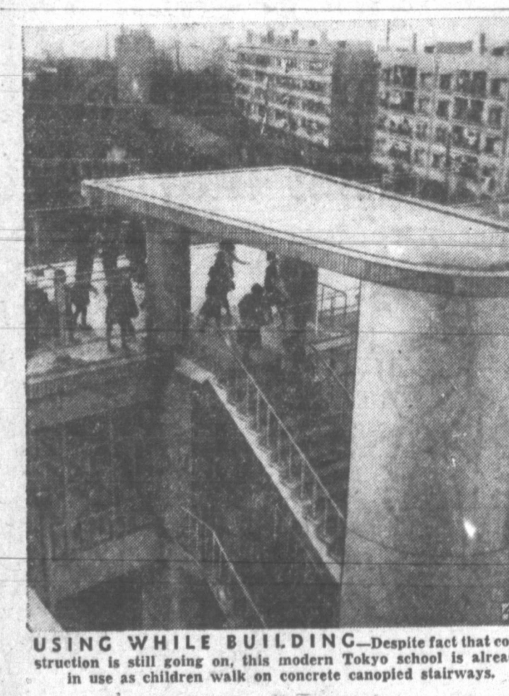
USING WHILE BUILDING - Despite fact that construction is still going on, this modern Tokyo school is already in use as children walk on concrete canopied stairways.
