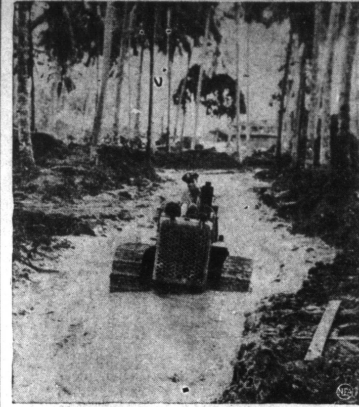
Before long a smooth hard road will replace this palm-fringed river of mud at a U. S. base in New Guinea. Scaabee driving a tractor is one of scores of Navy Construction Battalion workers now building roads, docks and other installations in jungle area.
