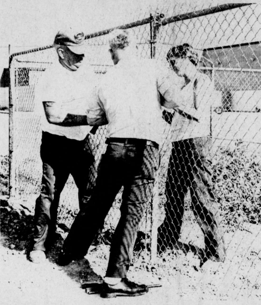
FENCE COMPLETED--From left, Wayne Holmes, Claude Holmes and Mrs. Wayne Holmes are completing the final section of the large cyclone fence that encloses the site of the miniature golf course to be constructed by the Muleshoe Area Youth Activities Committee Inc. Next on the construction list will be to construct the slab to house the concession/ticket/restroom building on the west side of the golf course.
