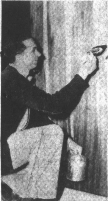
PASTOR HELPS —The Rev. M. D. Smith joins members of his church in building the new addition. He is shown above shelving the door to his new study. (News Photo and Engraving)
