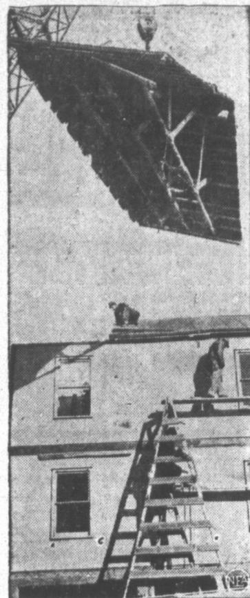
Crane lifts section of roof from temporary home at FHA's project in East Hartford, Conn.
