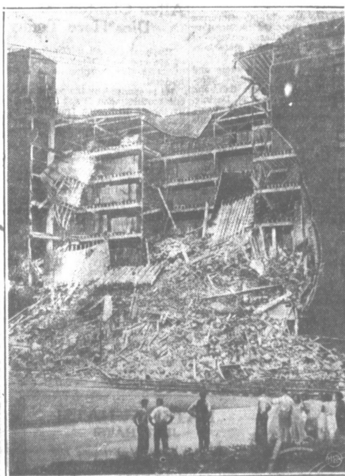
Here is one relief problem that presents a colossal job of "digging out from under." In the collapse of a seven-story Chicago warehouse where the government had stored hundreds of tons of food for the needy, the structure was packed to capacity, as the shelves along the wall still standing show. When one wall crumbled, thousands of barrels and sacks of foodstuffs and boxes of canned goods were buried in the debris. A fire several years ago is believed to have weakened the walls and vibration of switch engines nearby to have caused the collapse.
