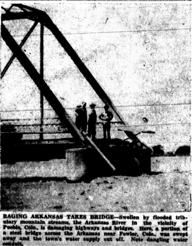
RAGING ARKANSAS TAKES BRIDGE—Swollen by flooded tributary mountain streams, the Arkansas River in the vicinity of Pueblo, Colo., is damaging highways and bridges. Here, a portion of a steel bridge across the Arkansas near Fowler, Colo., was swept away and the town's water supply cut off. Note dangling water conduit.
