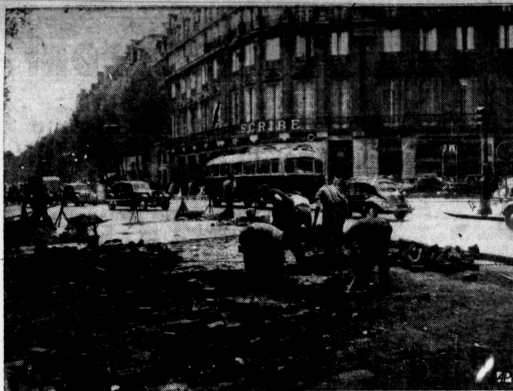
PARIS TEARS UP WOOD PAVEMENT—Workers take up wood blocks on the Boulevard des Capucines, Paris, to replace them with bricks and asphalt, safer for autos when wet.
