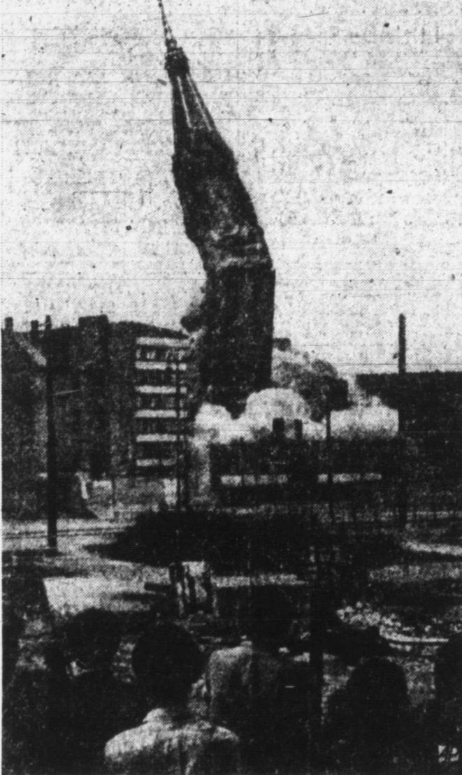
CHURCH STEEPLE BLOWN UP —The steeple of St. George's Protestant Church is blown up by an East Berlin demolition squad after Communists declared it a safety hazard.
