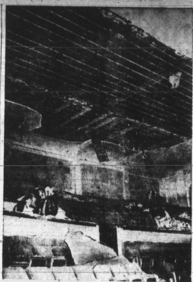
IT BROUGHT DOWN THE HOUSE —Firemen in Redwood City, Calif., look about the balcony of a theater where a movie called "The Gimpfinger" literally brought down the house. Several persons were injured when a large part of the ceiling collapsed. One woman jumped from the balcony and broke both legs.
