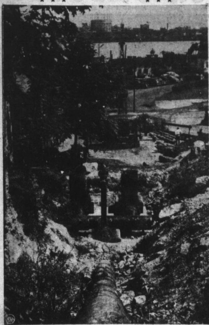
HEADING FOR THE RIVER — Other end of the gas pipeline you see here at Edgewater, N. J., is in Corpus Christi, Texas. Soon it will reach across the river to New York, in the background.
