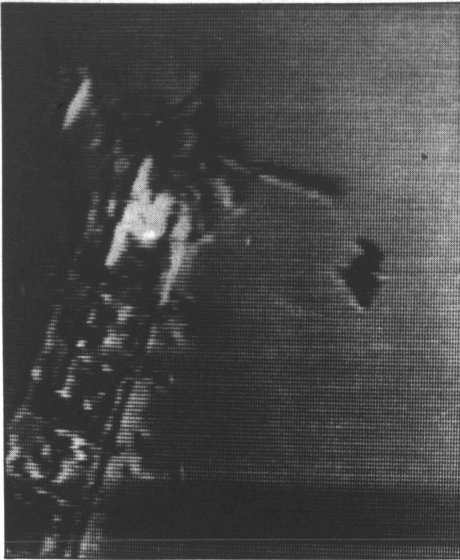
One of five people who died when a radio tower collapsed, falls to his death Tuesday near Missouri City. Project engineer Andy Hudac filmed the accident with his home-
