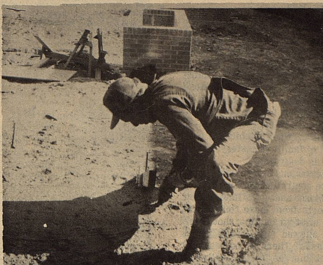
A concrete finisher touches up the floor being poured in the patio. The patio will contain benches, tables and shrubbery.
