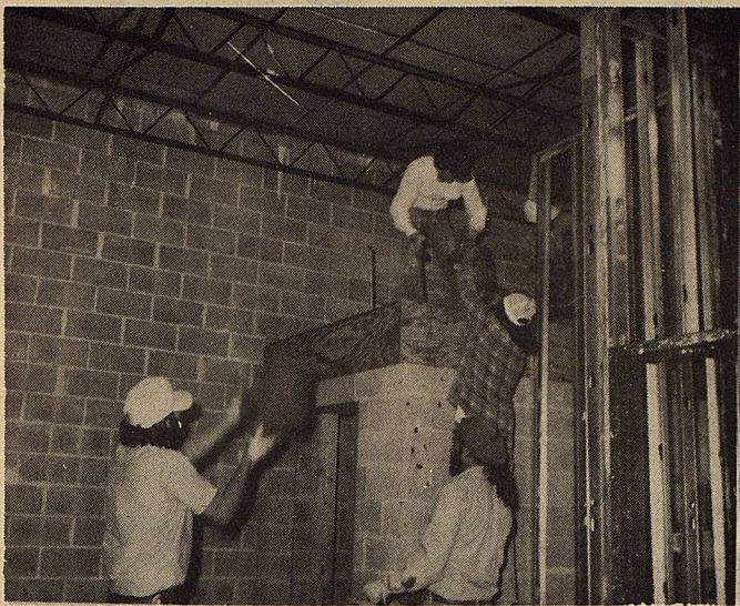
A team bucketing concrete to the roof of the vault in the new school addition.
