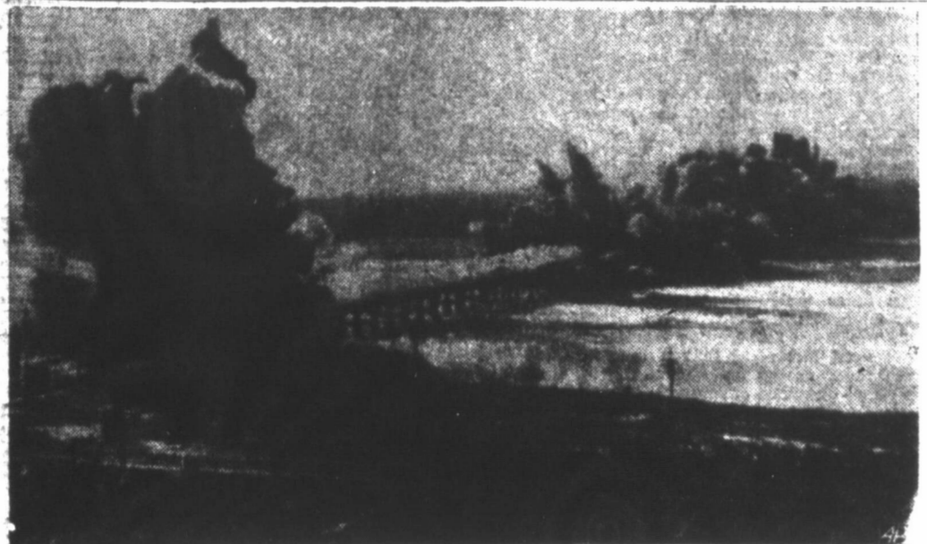
ONE BRIDGE THE REDS CAN'T USE—Demolition charges set by United Nations engineers blow a Songchon River bridge at Hamhung sky high Saturday as Allied forces withdrew from the north-east Korean industrial city ahead of hard-pressing Chinese Reds. (AP Wirephoto)
