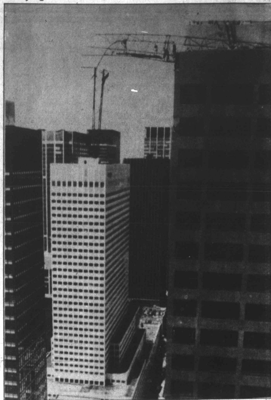
Workmen climb 43 stories over Manhattan as they work to secure a dangling section of a construction crane which collapsed
