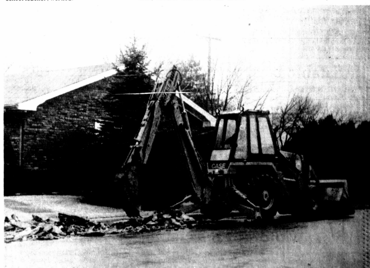
STORM SEWER PROJECT BEGINS. This backhoe begins ripping up the pavement at 22nd and Charles to make way for a mammoth, five foot cast-in-place concrete storm sewer pipe that will handle drainage in connection with improvements to State Highway 70. The
