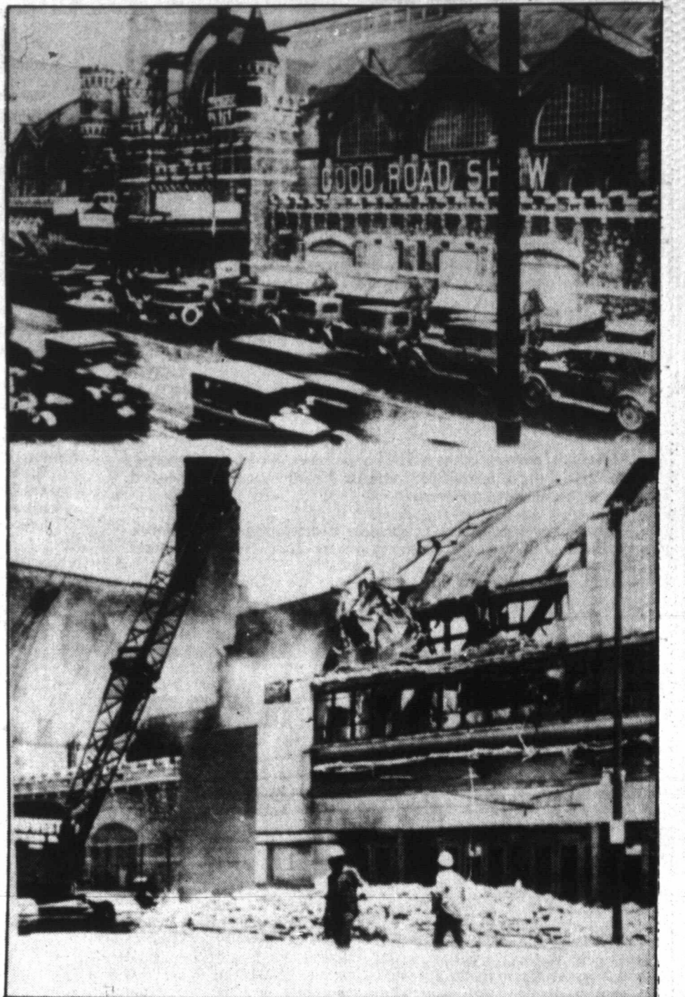
TUMBLING DOWN. The Chicago Coliseum, opened in 1900 and the site of numerous presidential conventions, sporting events and other entertainment, is now falling to the wrecker's ball, bottom, for development by a Chicago corporation. The Coliseum is shown in its heyday, top, circa 1927. (AP Laserphoto)
