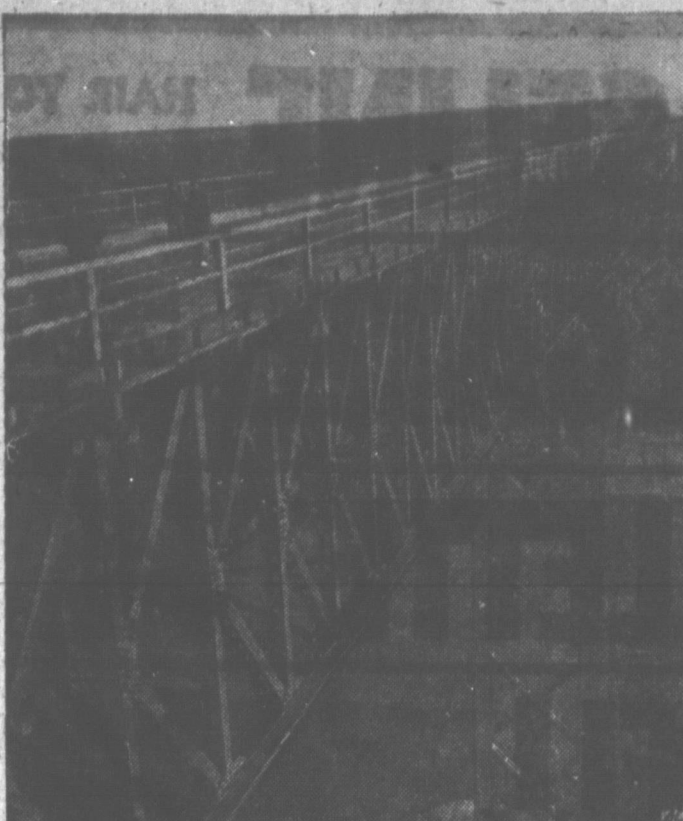
NEW GERMAN SPAN — Workmen finish the new surface of the bridge across the Larn Valley near Limburg, West Germany, destroyed by retreating Germans in 1945. It connects autobahn traffic from southern Germany with the industrial Ruhr.
