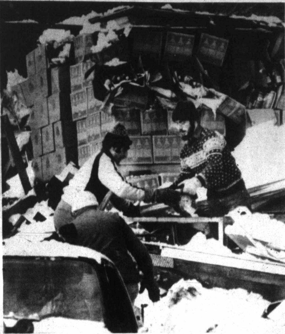
BROUGHT DOWN THE HOUSE. Domnic Arceci, left, and his son, Gary, handle the contents of a beverage company warehouse at Jaffrey, N.H., that collapsed under heavy snow.
