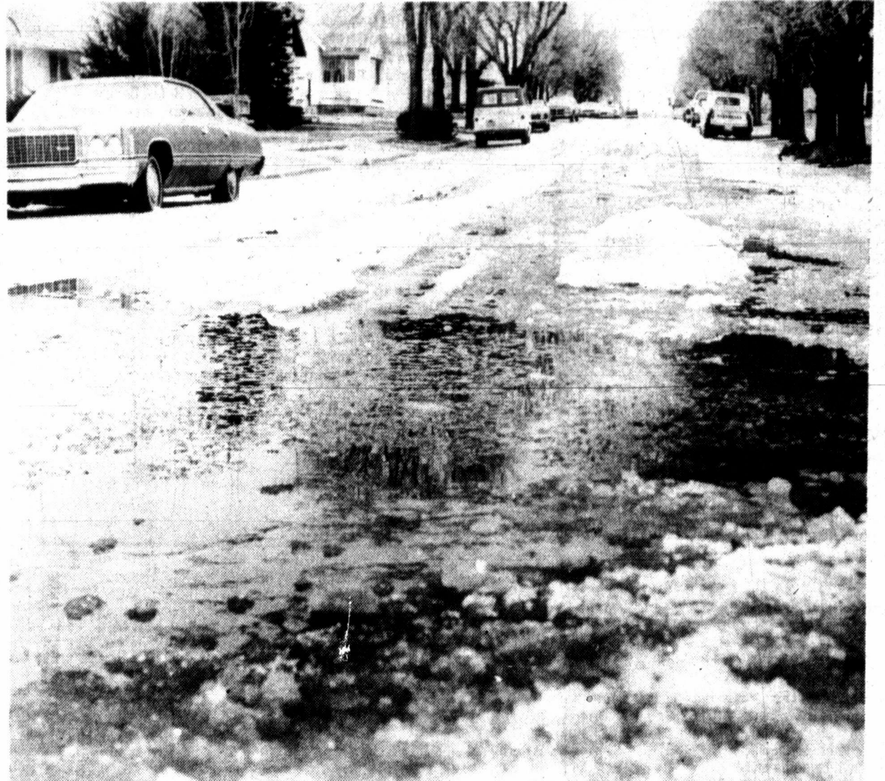
AN OVERNIGHT WATER MAIN BREAK on Francis and Somerville Streets caused an unexpected buildup of ice in the 500 to 900 blocks of Frost Street. Early morning motorists were left wondering where it all came from as they slowed down to miss the chunks of floating ice. (Staff Photo by John Wolfe)
