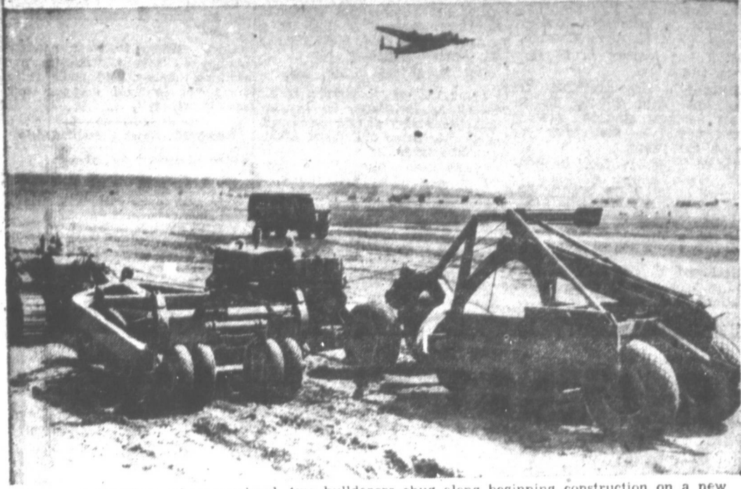
As an airlift plane wings overhead, two bulldozers chug along beginning construction on a new runway at Gatow Airfield in the British sector of Berlin. With Soviet-U.S. negotiations under way to lift the Russian blockade of the city, occupation officials hope the urgency for more landing strips will disappear, but they're taking no chances.
