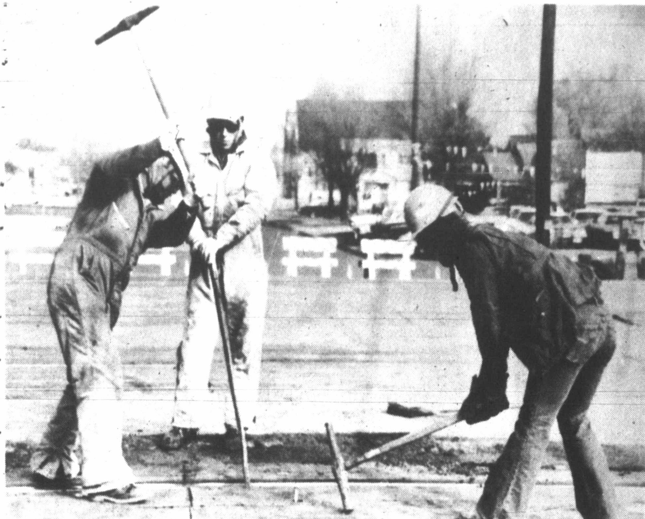
WORKING ON THE RAILROAD. Santa Fe Railway employees Jesse Cuellar, left, Kenny Bacon, center, and Gary Patin are rebuilding the railroad crossing at Starkweather Street. The intersection is one of three track intersections Santa Fe will be improving in the near future. (Staff Photo by Skyler Chapman)
