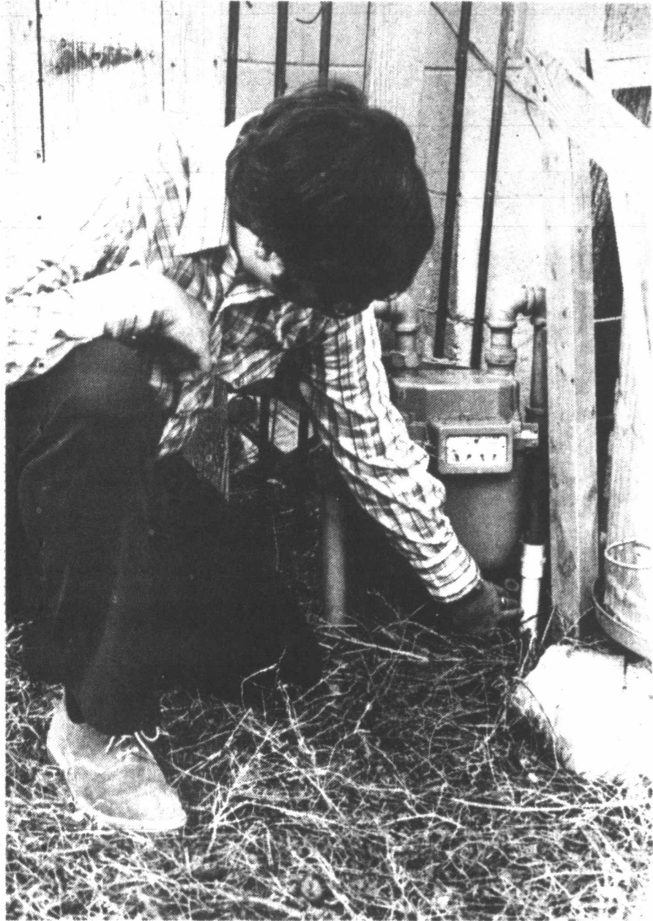
EXPLOSION HAZARD. City Building Inspector Steve Vaughn points to a plastic natural gas "riser" located behind a residence in the 1100 block of Christine. Vaughn says the plastic gas lines are "time bombs" which could explode if struck by a passing garbage truck or other vehicle. Officials of Pioneer Natural Gas Company say service will have to be discontinued at residences with the plastic lines unless the lines are replaced with black steel. (Staff Photo)
