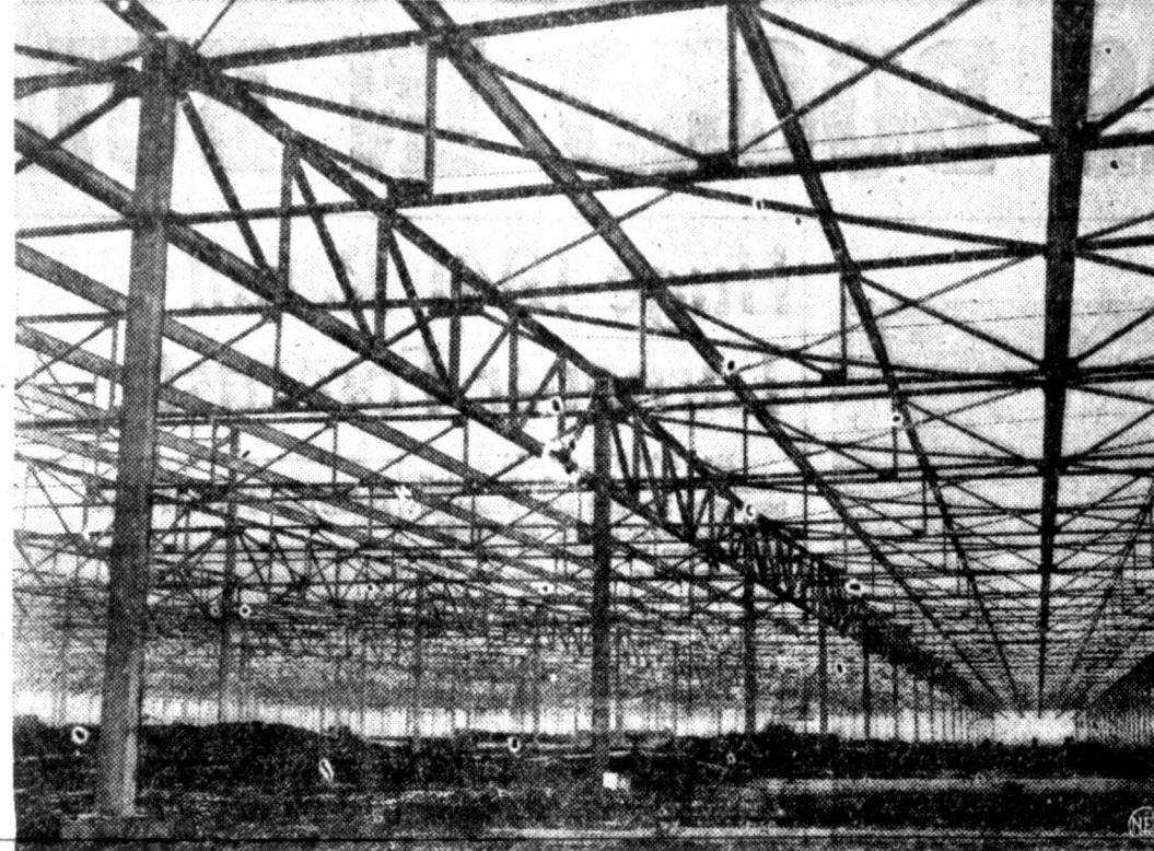
This view of the structural steel work on the North American plant gives an idea of the immensity of the building. Tiny speck in right extreme background is a man.
