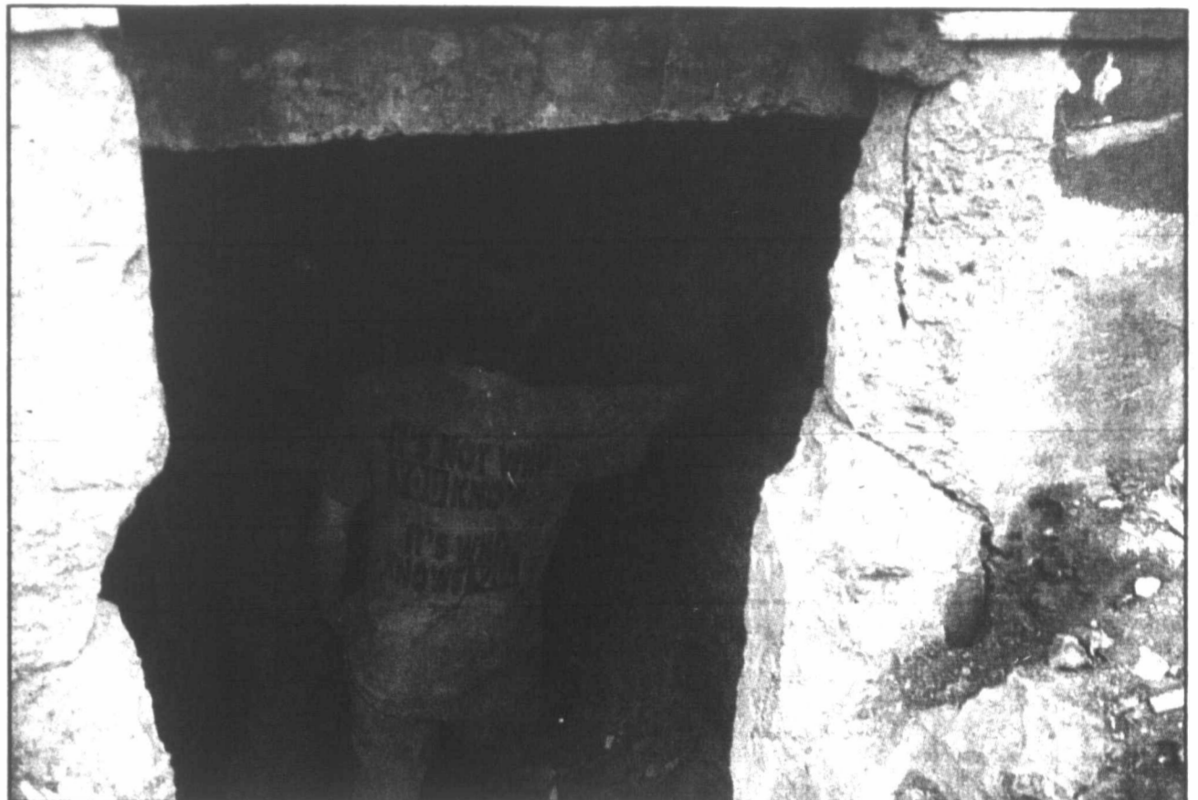
Workers from C and K Contractors pound through a basement wall this morning at 403 N. Ward. Police hope to find the remains of a man supposedly murdered and buried there in 1928.
