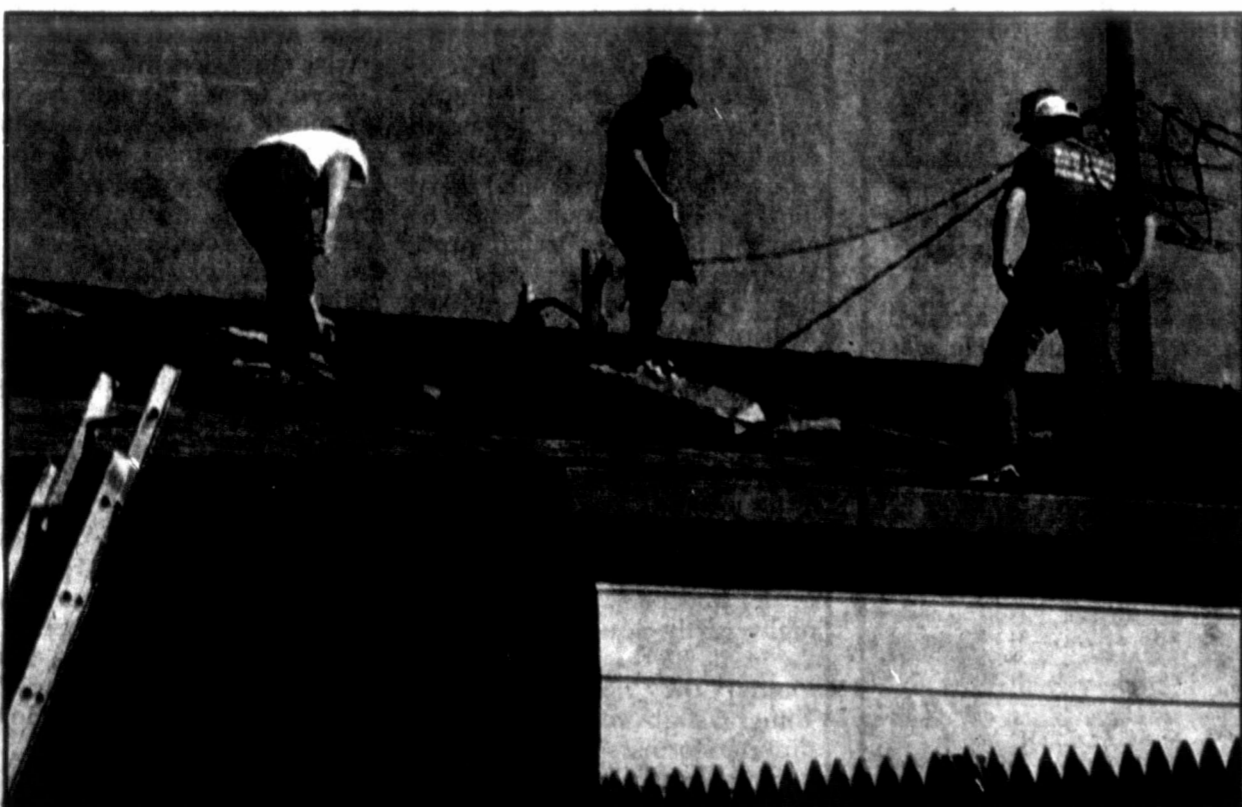
Jeremy Herndon, Rod Herndon and Brian Marsh work diligently under the hot sun reroofing a garage this morning on Dwight Street. The young men work with Roderick construction and were repairing Rick Marsh's garage roof.
