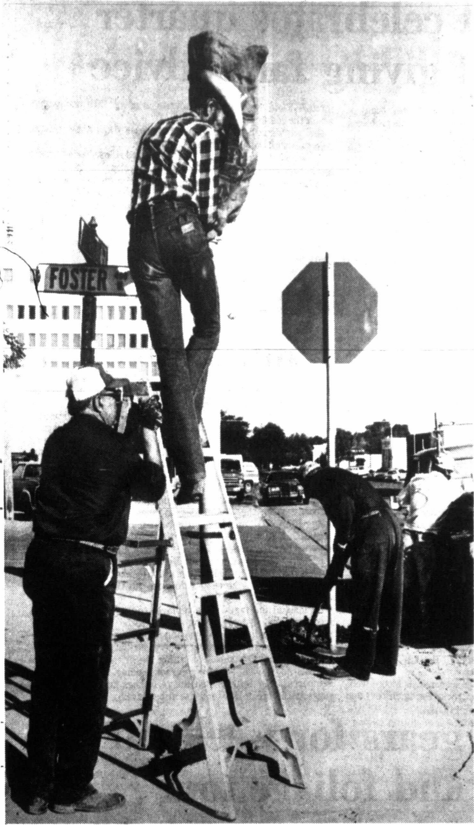
TRAFFIC EXPERIMENT. City of Pampa employees are shown here "bagging" the lights at the intersection of Foster and Somerville Street and installing stop signs for Somerville traffic Wednesday. The city hopes to gain public input before permanently removing the lights from the intersection. Employees are (from left) V. L. Hampton, Alfred Oxley, Leslie Edmondson and Alfredo Campos.
