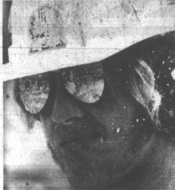
DUST RAISING PROJECT. Sand from the drilling he is doing coats the face and glasses of Pete Fowler, at work on excavation for the Tennessee-Tombigbee Waterway at Bay Springs, Miss. Fowler is drilling holes for explosive charges, to clear rock for the Waterway's middle canal section. This is part of the monumental task of tying together 12 river systems for the 253-mile project, which will extend from the Tennessee Valley to the Gulf of Mexico. (APN Illustration)
