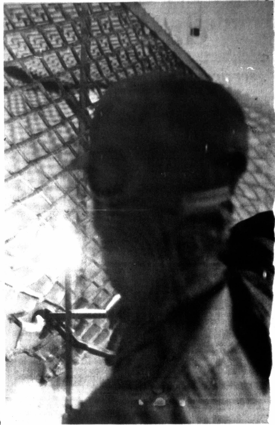
REPAIRING THE DAMAGE. City Maintenance Supervisor Robert Herring welds back the grill on the juvenile detention cell at city jail early today after the grill was damaged by two juveniles who escaped from the facility at 3:30 a.m. this morning. The two boys, ages 12 and 14, were apprehended by police at 5:26 a.m. after a high speed chase and a foot pursuit through city streets. (Staff Photo)
