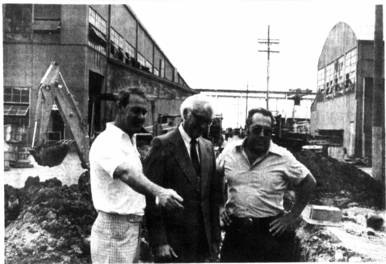
INGERSOLL-RAND OFFICIALS view preliminary work to the construction of a new $1 million office building at the Ingersoll-Rand Oilfield Products Company plant site west of Pampa. Above, Walt McFatridge, left, manager of manufacturing operations, points to work on a sewer line at the site. With him are William G. "Bill" Mulligan, center, of Wood Cliff Lake, N.J., executive vice-president of Ingersoll-Rand, and Vic Raymond, right, president of Ingersoll-Rand Oilfield Products Company. (Staff Photo)
