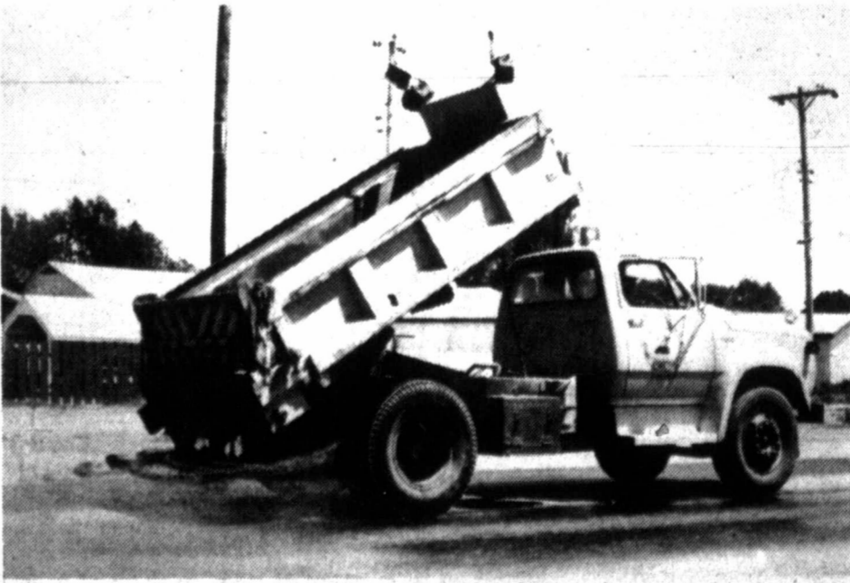
SAND IS BEING USED AS A TAR BLOTTER as trucks continue to work Pampa streets, sticky with tar as a result of high temperatures. The asphalt base of much of the street paving in the city has become tacky as rays of sun liquify the petroleum agent in the surface. (Photo by Ed Sackett)
