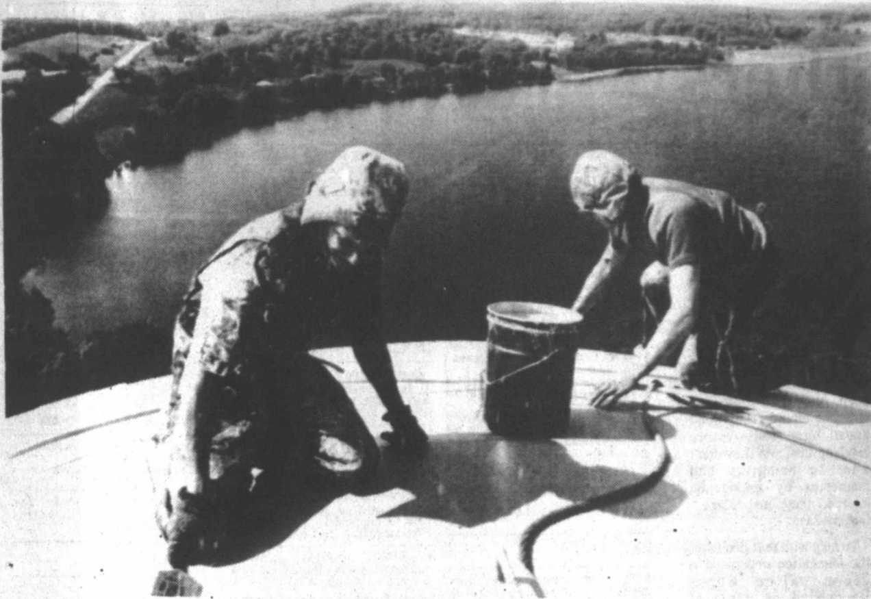
WORKERS HIGH ON A TOWER in Avon, Minn., like carnival workers, travel through rural areas each summer mystifying the locals with their daring tricks. The two on this 150-foot tower, though there to paint, couldn't help but admire the view, five miles in any direction. (AP Laserphoto)
