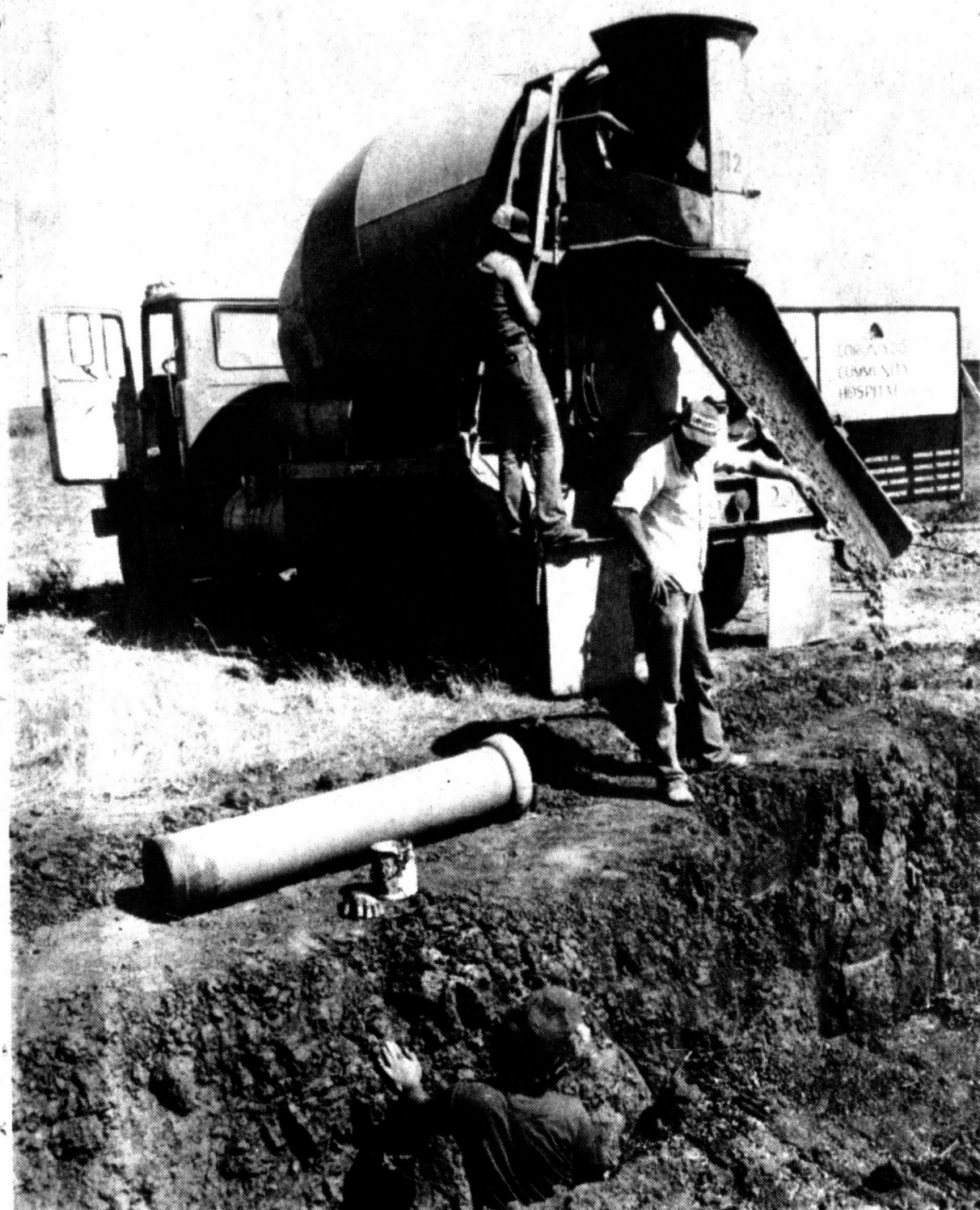
WATER AND SEWER LINES at the new Coronado Community Hospital site are being installed by crewmen of the Robert W. Taylor Construction Company, as the first step in construction of the new hospital. Preparing to pour the base for the lines are Jimmy Green, of Pampa, on truck; Richard Glover
