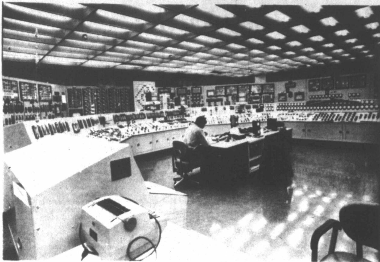
NUCLEAR SAFETY. The control room at Three Mile Island Nuclear Plant near Harrisburg, Pa., is said to be 10 years behind latest technology. This statement is credited to Harold Denton, NRC spokesman. (AP Photo)
