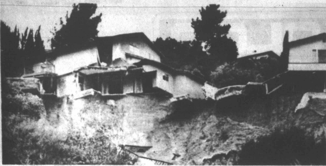
PRECARIOUS PERCH. The rear of the house at left hangs precariously over a section of a washed away hillside in Stone Canyon section of Los Angeles.
