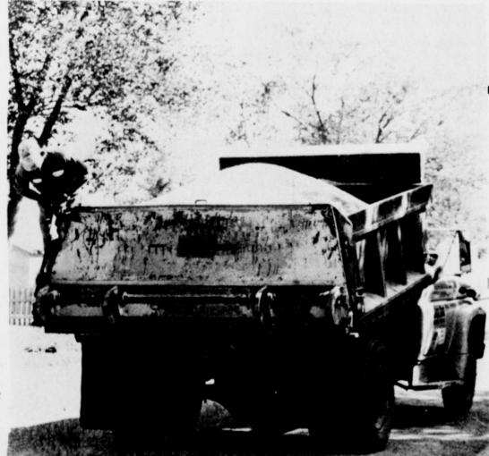
PAVING PROJECT -- Muleshoe streets -- 70 blocks or so -- have been given a "re-touch" job. Here's a Jake Diel truck covering one of the "bleeding" spots in the asphalt. (Journal Photo)
