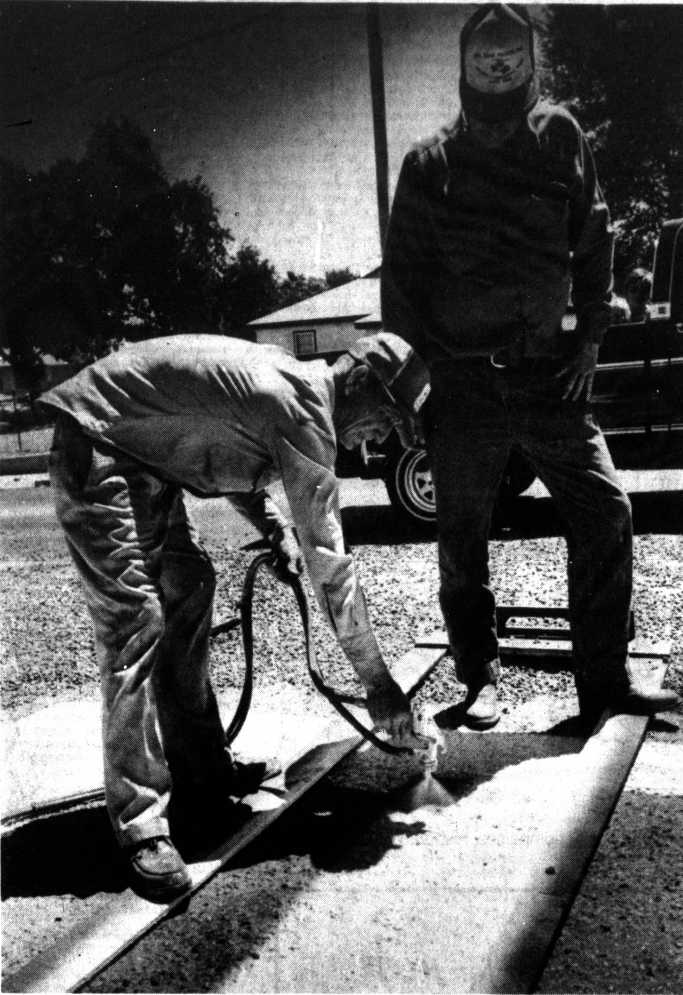
SCHOOL DAYS are less than two weeks away, so Pampa city crews are retouching crosswalks to make things safer for children who hoof it to class. These men were repainting the crosswalk at Perryton Parkway and 23rd Street Monday afternoon. (Staff photo by Gary Clark)
