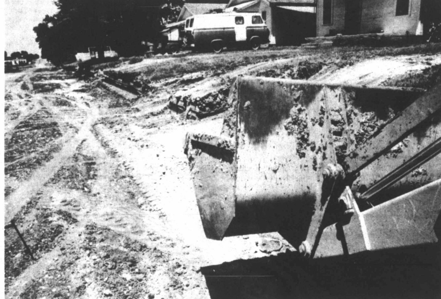
AN AMBITIOUS STREET-PAVING PROGRAM began June 18 in Wheeler. About 44 blocks will be paved at an estimated cost of $624,958.17. The work is being done by Lewis Construction Co. of Dumas, and is expected to take the rest of the summer. (Staff photo)
