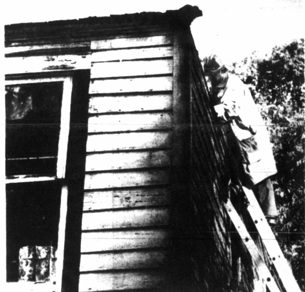
FIREMEN were called to this vacant East Browning Street garage apartment Friday evening to contain a blaze which broke out shortly after 6 p.m. The cause of the fire is unknown. Heavy damage was reported to the roof and side of the apartment.
