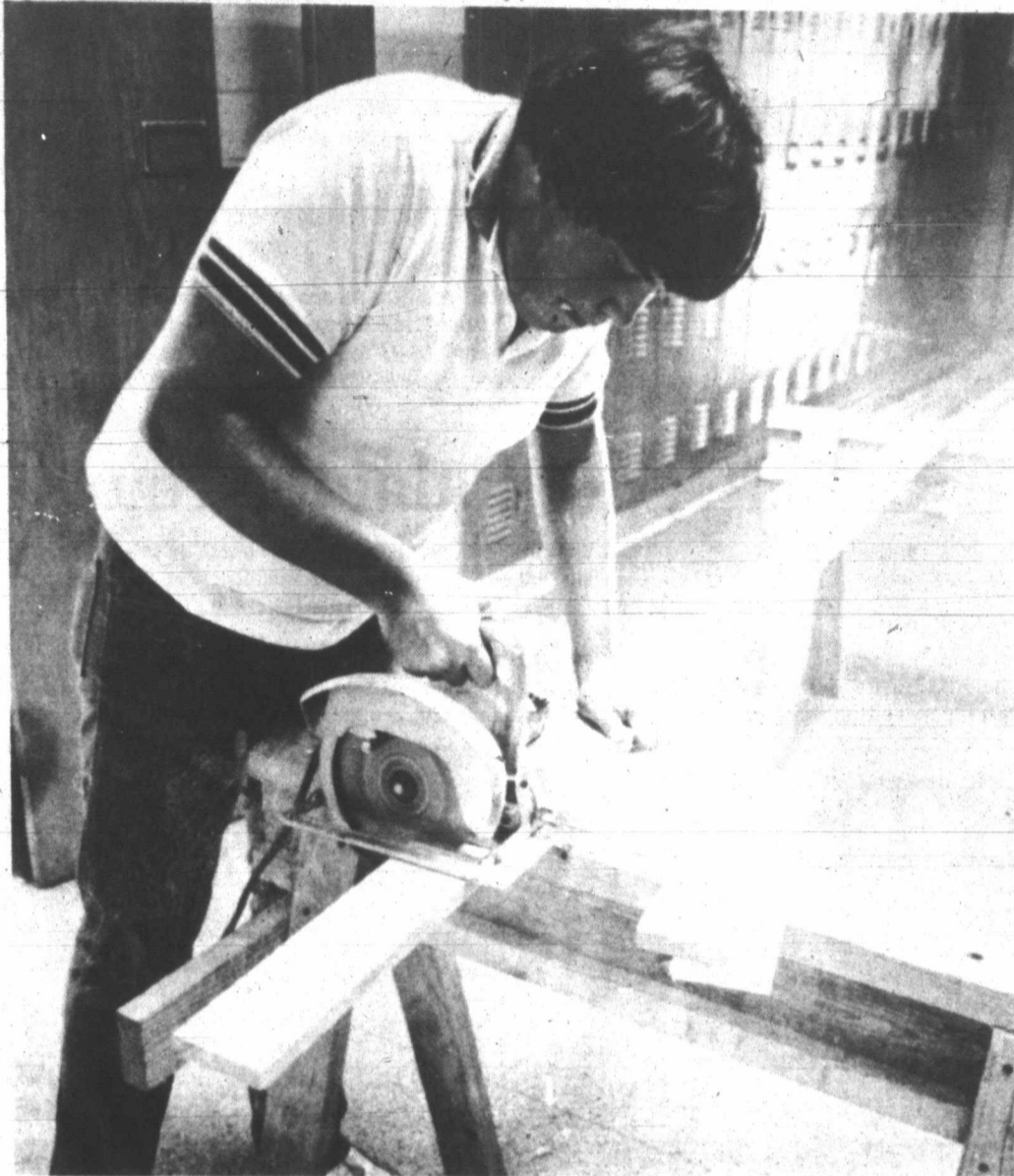
RANDY CARPENTER cuts wooden segments, which will be the base for the panelling to be placed in his alma mater, Pampa High School. According to the construction foreman, Dave Rawlins of Lubbock, the work for this part of the renovation work should be done before school starts. The crew, hired by the contractor - Monterey Construction Co., began Monday after Rawlins surveyed the project over the weekend. The panelling was expected to arrive Friday. The Monterey Co. may be contracted to finish building the concession stands at the football field. The building trades class began their construction, but had difficulty completing them because of weather problems. (Courtesy photo by Ed Sackett)
