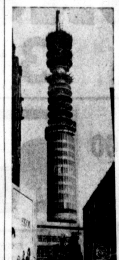
TOWERING PROGRESS —Beginning to take shape, the general post office television and radio-telephony tower gradually nears its completed height. The tower, under construction in Bloomsbury, West Central London, now stands 477 feet. It will be 619-feet-high when finished.
