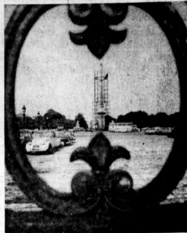
CONSTRUCTIVE FRAMING —Viewed through the ornate fence near the Place de la Concorde, the Luxor Obelisk of Paris looks like a rocket; it's being cleaned.
