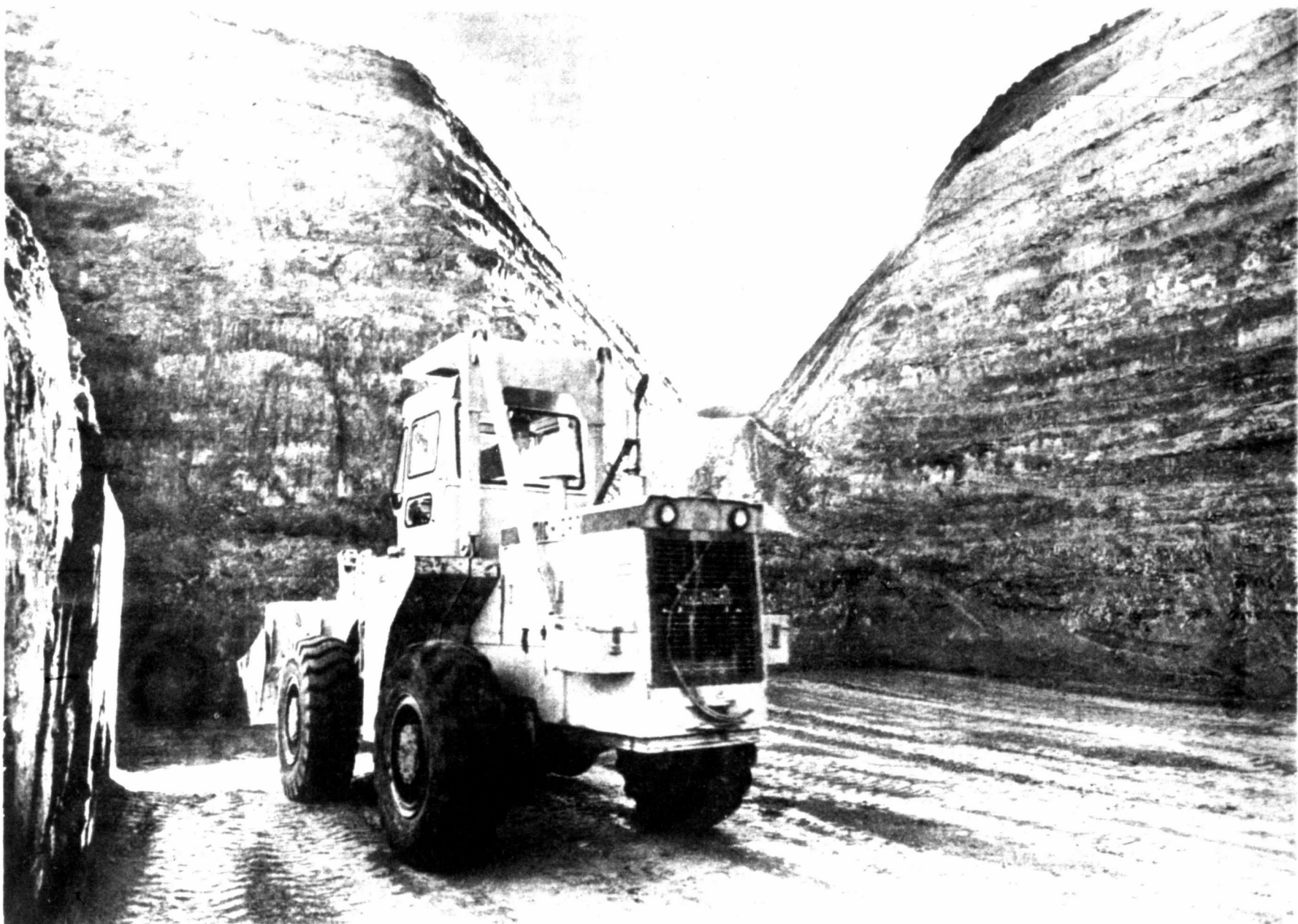
Work is progressing at Celanese on the company's energy conversion program. This massive pit will provide underground storage of coal to be burned at the rate of 1,600 tons
